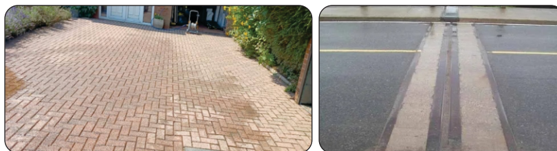
Figure 10.7 Gaps in concrete surface of road
